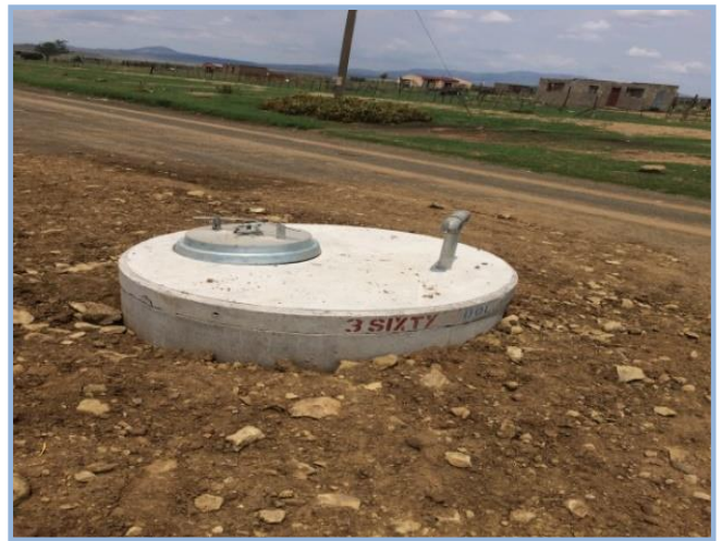
Concrete manhole: air-valve
