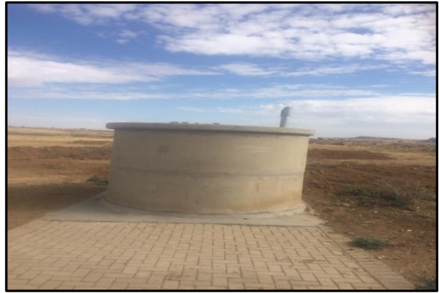
Air-valve concrete rings
